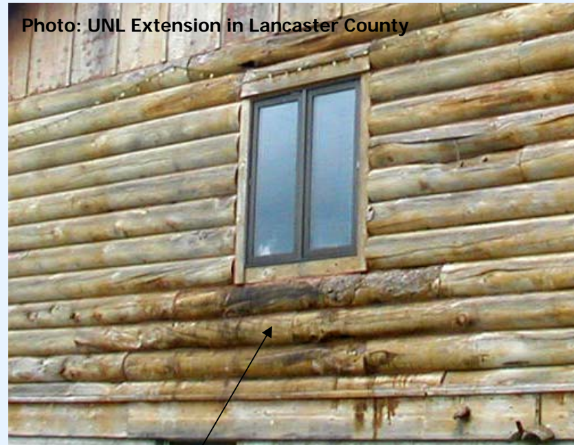
Discolored area below window Indicates moisture damage
