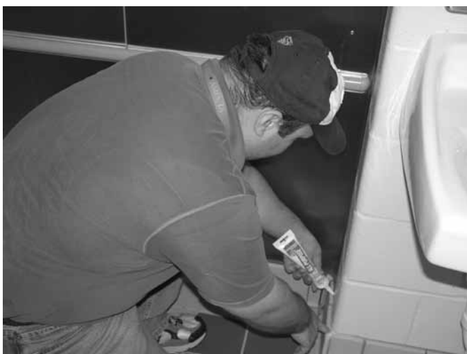
Sealing holes is a good example of habitat modification and exclusion as it reduces available hiding places for pests.
