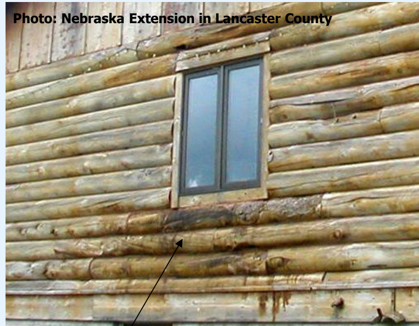
Discolored area below window Indicates moisture damage
